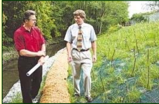
Anthony Marrocco '66 left, and Chief Engineer Keith Graboske examine the geo-web, a system of native plants, grass, and "live sticks" - tree stock that will grow into the bank to make it more stable
